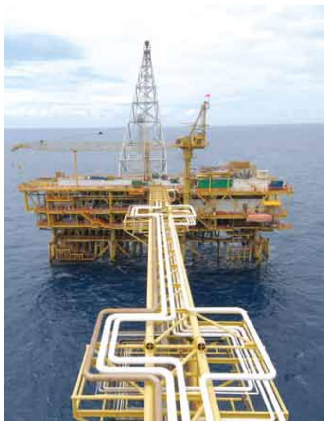
The Angsi project is the first Chemical EOR offshore pilot project in the region
