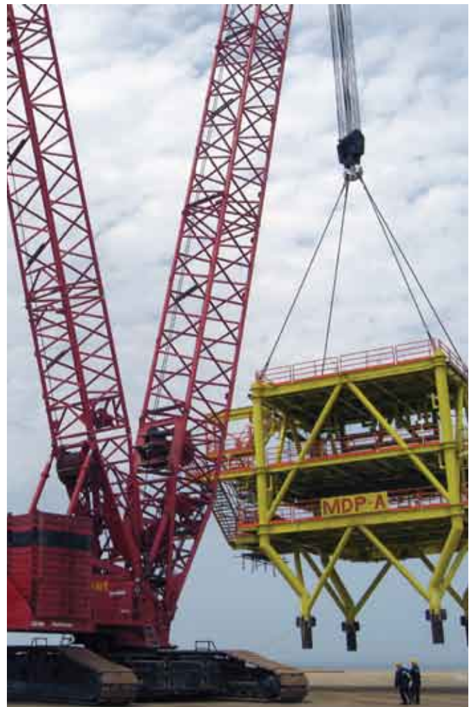
Magtymguly Drilling Platform - A (MDP-A) topside in Turkmenistan being offloaded from the fabrication area to the transport barge for offshore installation in the Caspian Sea
